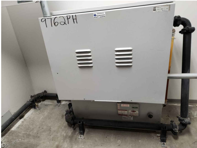
LOBBY ELEVATOR CONTROL ROOM - HYDRAULIC POWER
