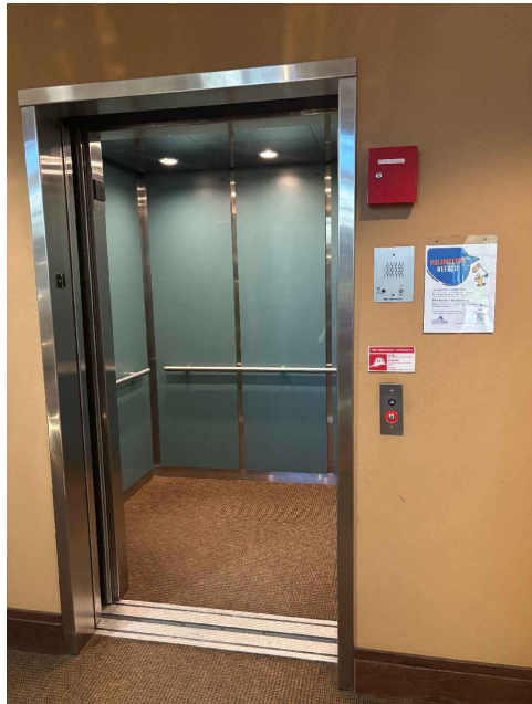
LOBBY ELEVATOR LOWER LEVEL - FRONT VIEW OPEN
