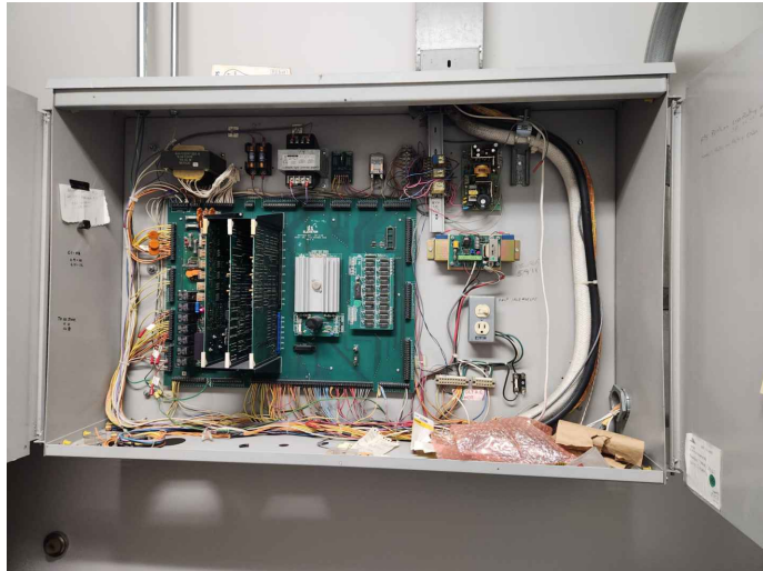
LOBBY ELEVATOR CONTROL ROOM - ELEVATOR CONTROLLER
