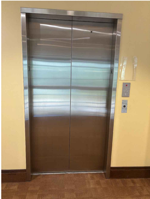
LOBBY ELEVATOR UPPER LEVEL - FRONT VIEW CLOSED
