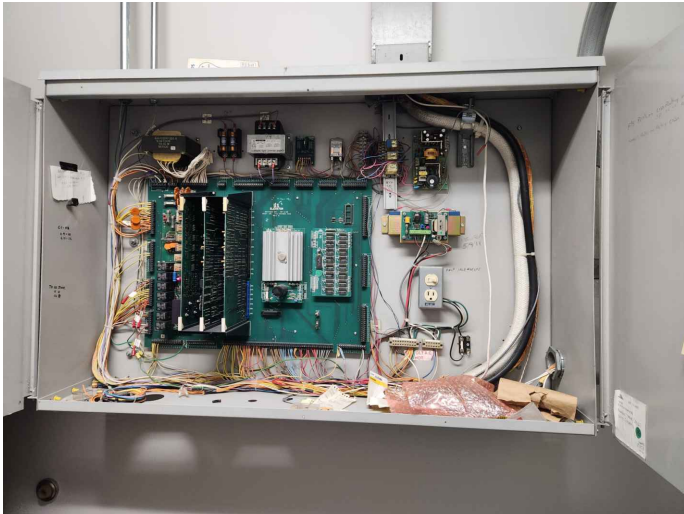
LOBBY ELEVATOR CONTROL ROOM - ELEVATOR CONTROLLER
