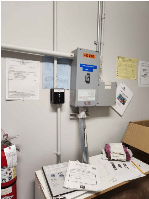
LOBBY ELEVATOR CONTROL ROOM - ELECTRICAL BOX
