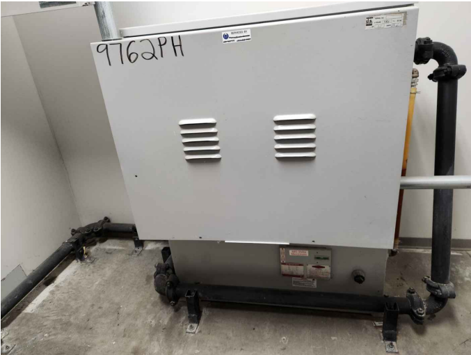
LOBBY ELEVATOR CONTROL ROOM - HYDRAULIC POWER
