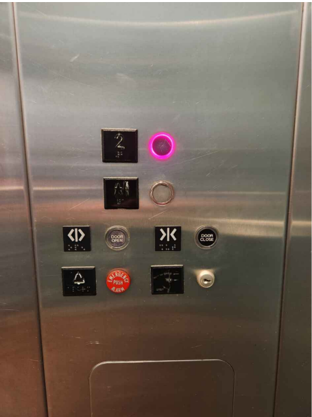
LOBBY ELEVATOR LOWER LEVEL - FRONT VIEW OPEN
